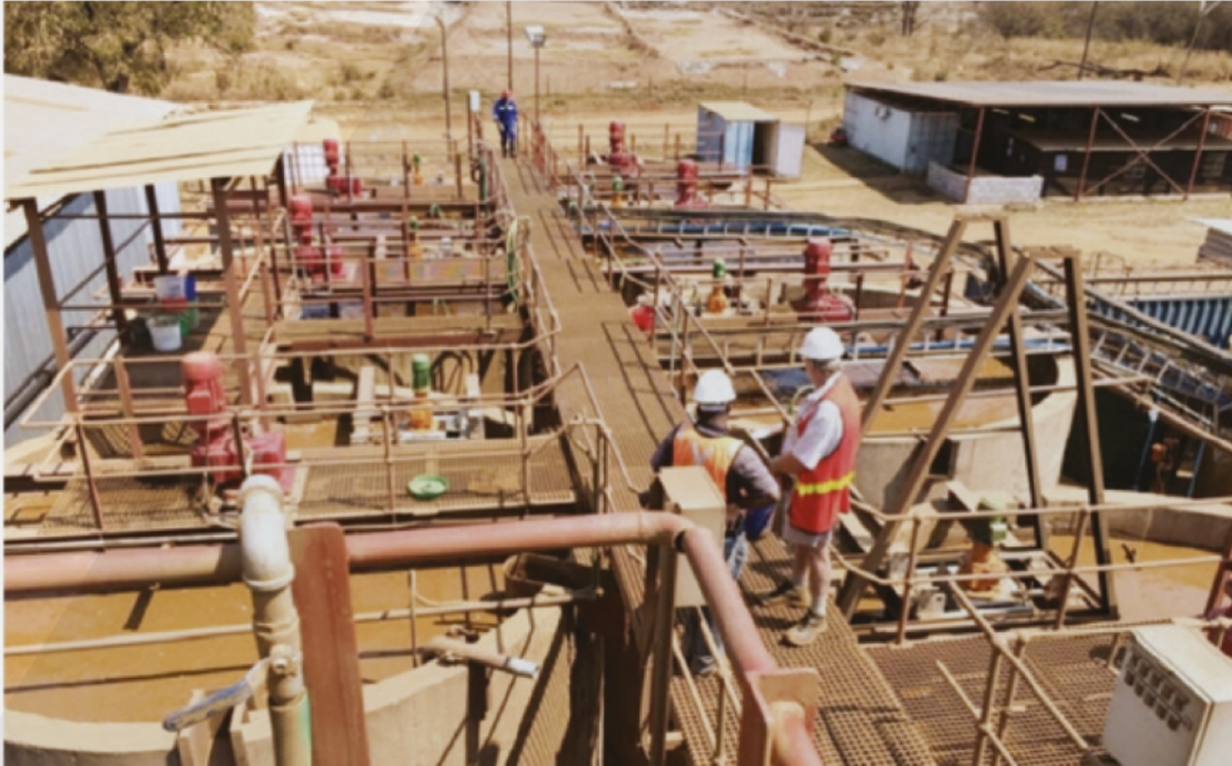
Eureka Mine has constructed new leaching tanks as part of the new gold processing plant.
